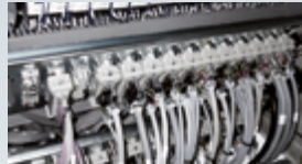
Solutions inside the control cabinets
